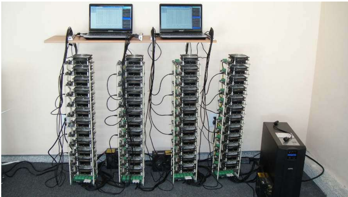
Figure 5.8: A home-built rack of FPGAs. Although you don't see the cooling setup pictured here, a rack like this would need a cooling system.
